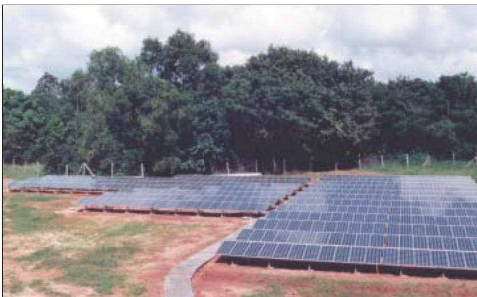
Figure 1: Matrimandir solar PV power plant.
